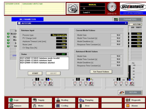
Fig. 20 Operator's panel window view – PID temperature regulator.
