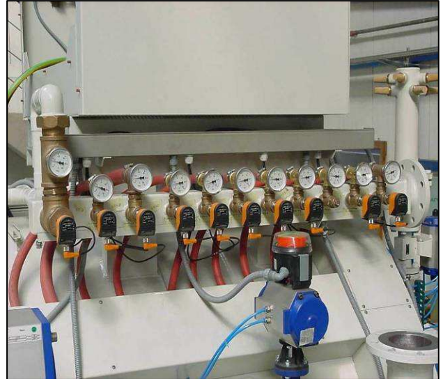
Fig. 19 Cooling water installation – main manifold.
